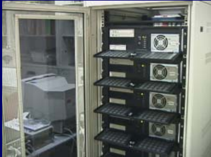
PC units mounted in a 19" rack
